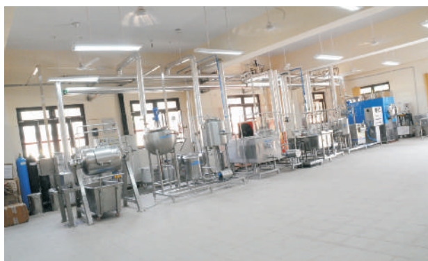
Milk and Milk Products Processing Plant Installed at BHU, Varanasi
