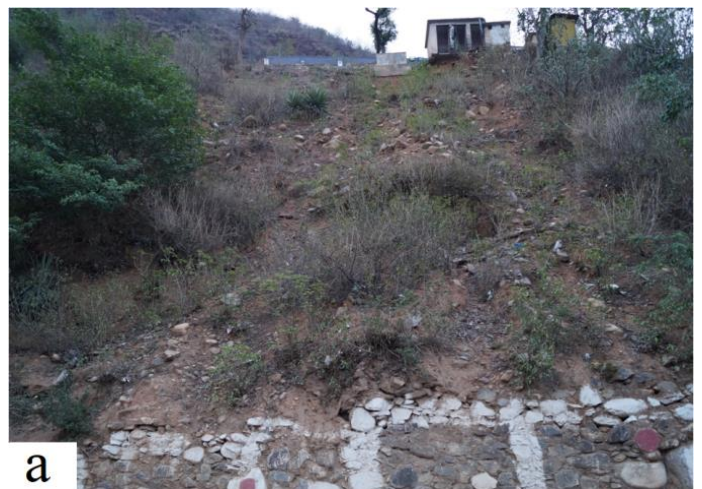
Fig.11 a. Photograph shows that the materials below the foundation of toilet, GGIC, Devprayag has eroded due to L_3 landslide.
