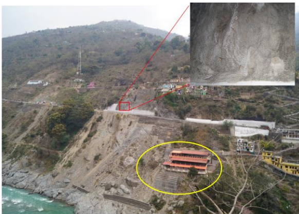
Fig. 9. Photograph shows L_1 landslide after treatment in 2018. A house marked by ellipse is still subsiding.
