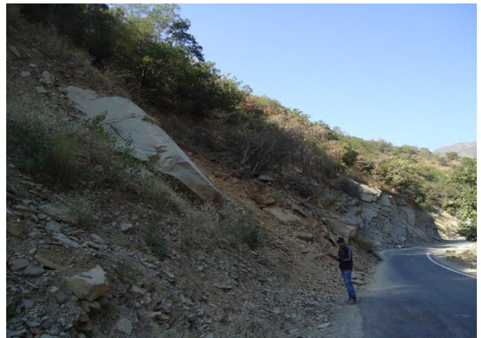
Fig. 13. Photograph shows debris slide of L 5 landslide.
